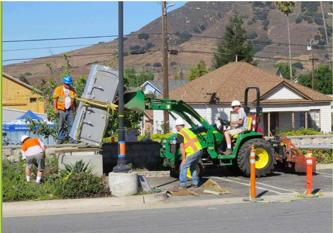
Museum members help erect the base for the Semaphore Signal Street Sign that will announce our location to all passersby. We hope to see it in place before the Central Coast Railroad Festival.
