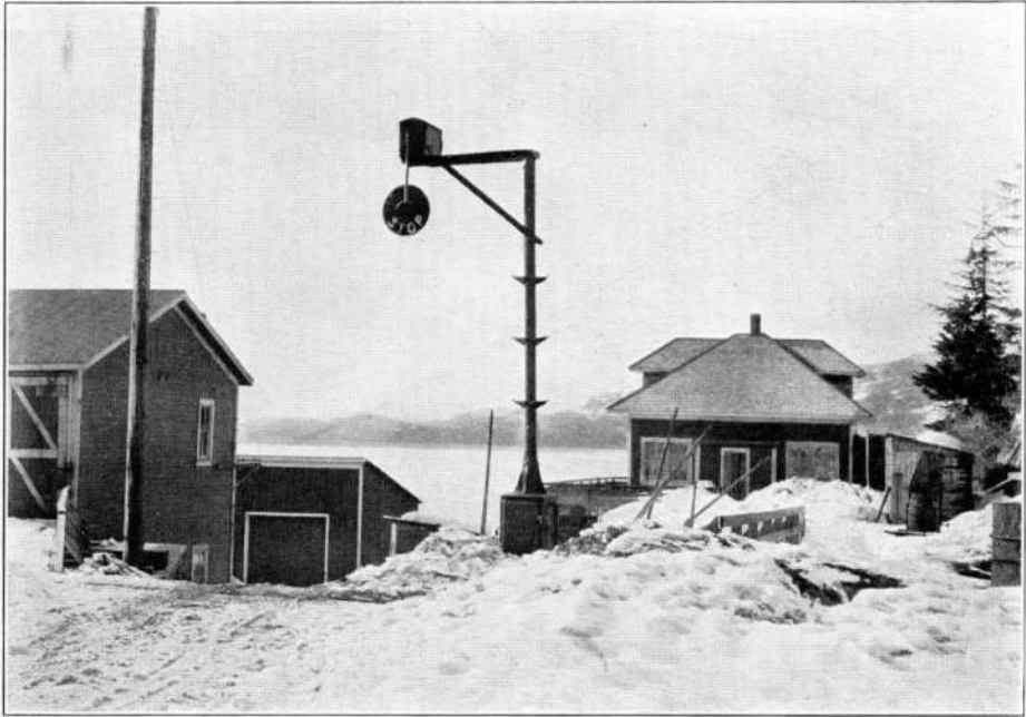
Installation of Magnetic Flagman (two position, lower quadrant), on the Copper River & Northwestern Railway at Cordova, Alaska.
