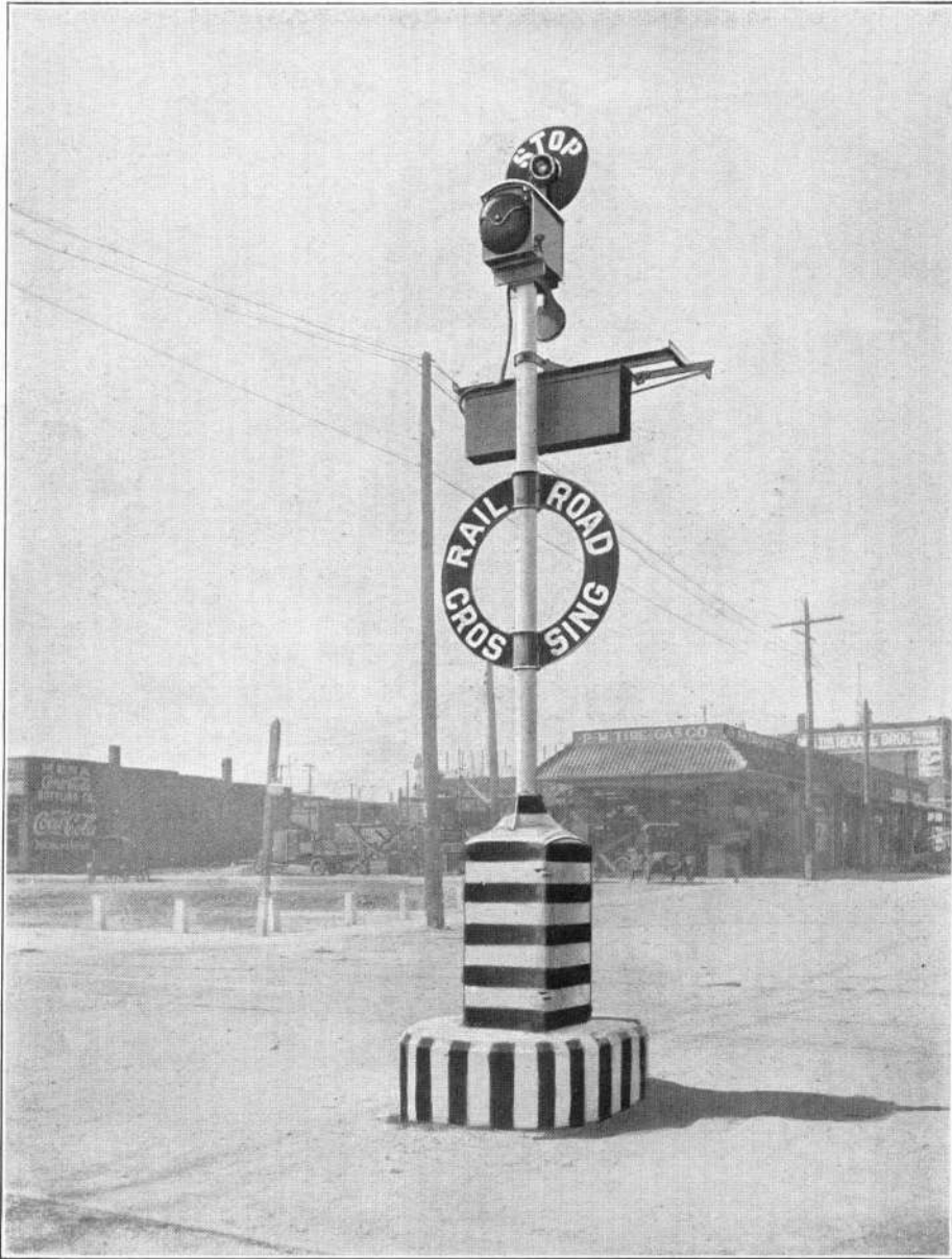
Center of Street Installation of Magnetic Flagman (two position, upper quadrant, with "Out-of-Order" attachment), on the Kansas City Southern Railway.
