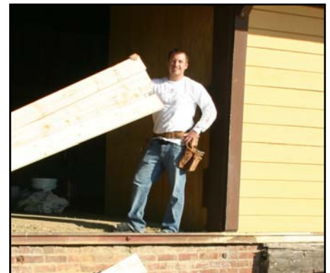
Ryan McKinley of RK Builders, Inc. supervising the unloading the trusses at the freighthouse on February 1st.
