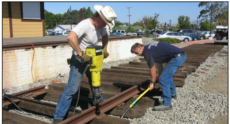
Brad "John Henry" LaRose drives spikes while Ted "Gandy Dancer" Van Klavern levels the rail on the display track in front of the Museum building.
